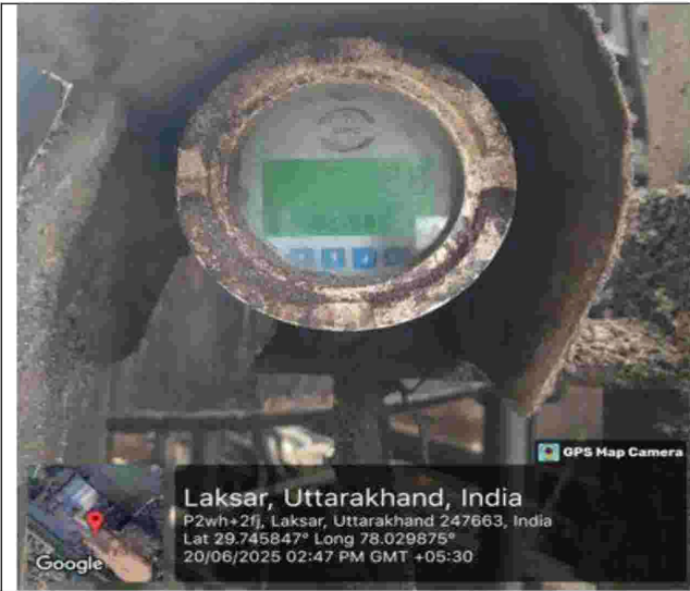
Flow meter installed at Feed to Old Spray Dryer
