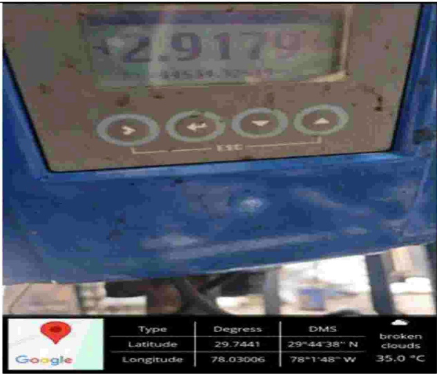
Flow meter installed at Feed to New Spray Dryer
